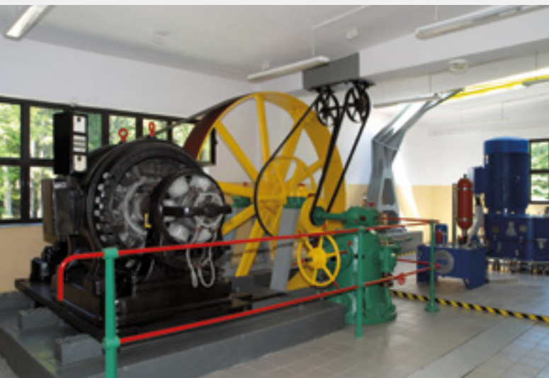
Poganice - Hydroelectric power station | Photo: L. Duchnowicz
